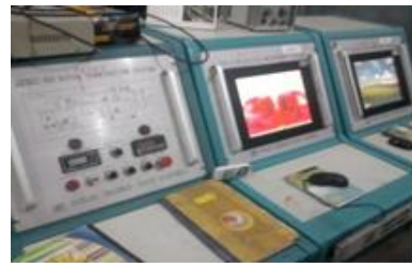
Fig 8: PD testing Set up panel with HV testing and PD calibrator.
