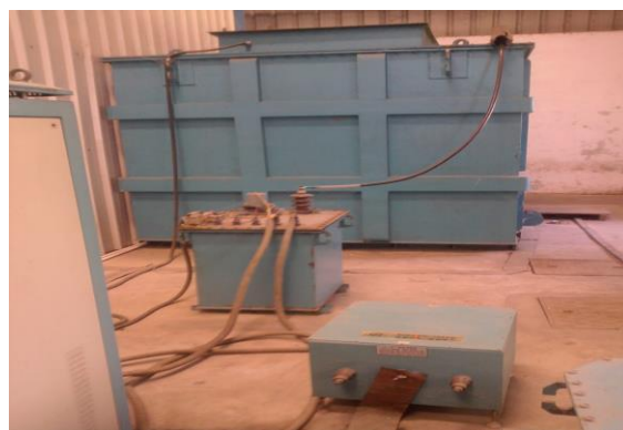
Fig 4: Resonance (LVDT) Transformer With Excitation Transformer
