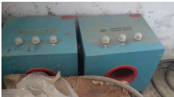
Fig 1: Cable Heating Current Transformer
