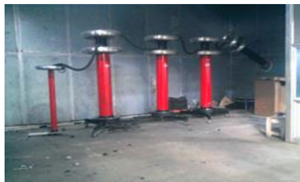
Fig 5: PD HV Resonance Set Of Transformer, PI Filter
